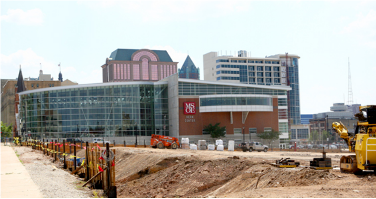
Excavation begins for development along the former Park East freeway. Photo Credit: City of Milwaukee
