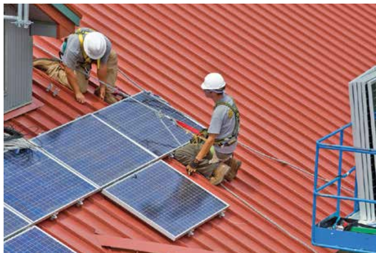
Photo 7: rooftop solar photovoltaic installation (Credit: Wayne National Forest)
